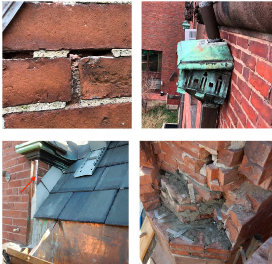
Examples of sections in need of repair Images courtesy of Foster Architecture
