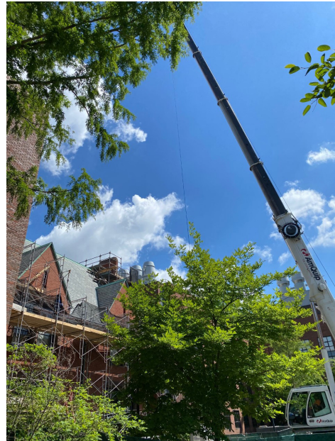
The large crane used during the construction Image Courtesy of Genevive Tocci
